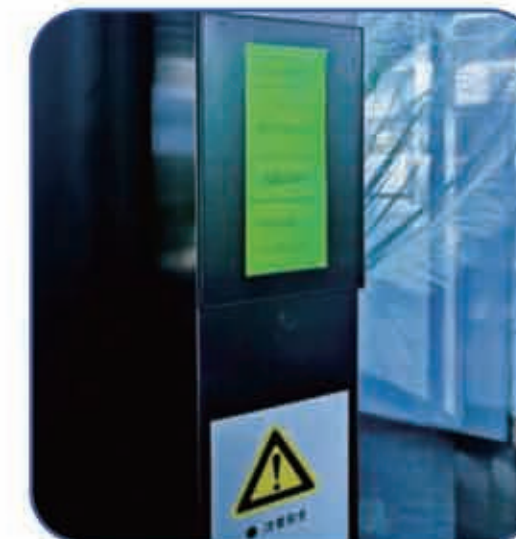
Control panel of revolving door
