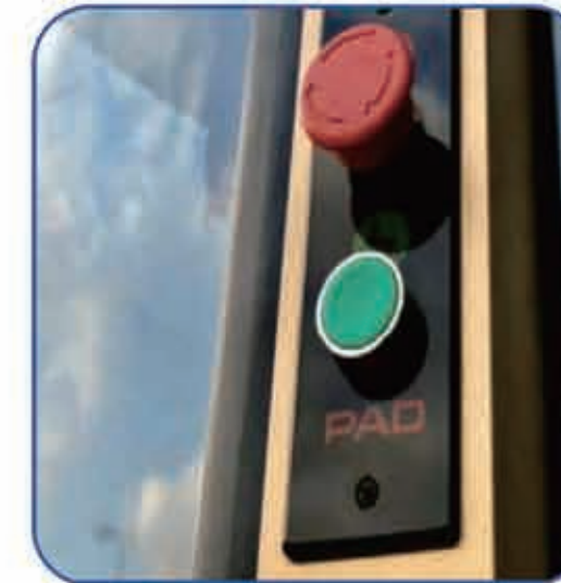
Start stop button of revolving door
